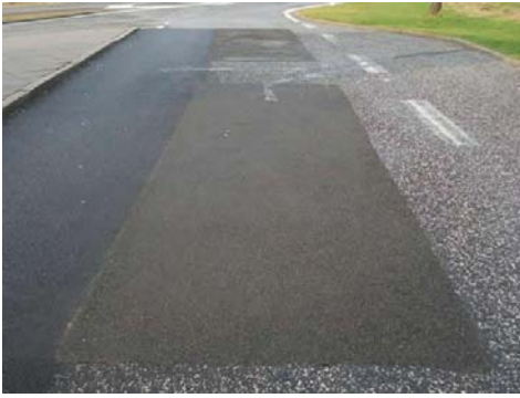
The two PERS test plates on the parking area along the Holbaek highway in Arnakke, Denmark.
