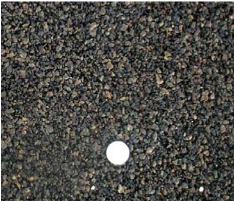
Macro view of the PERS surface on the test plate built in Arnakke in October 2011
